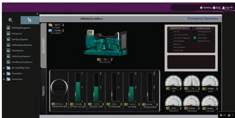
Figure 4: In this example, a variety of equipment points, trend settings and display options are shown for a single piece of equipment. Courtesy: SmithGroup
